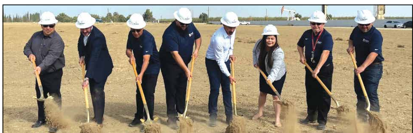
Breaking ground on Shafter's new $30 million sports complex. From left are board members Fortino Valdivia and Nelson Salinas, project consultant Gilbert Garcia SRPD District Manager Phillip Jimenez, The Wonderful Company's Andy Anzaldo, and board members Cristina Camacho, Gary Rodriguez and Amando Chavez.
