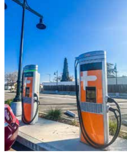
Two new Level 3 Stations located at 719 F St in Wasco, CA
